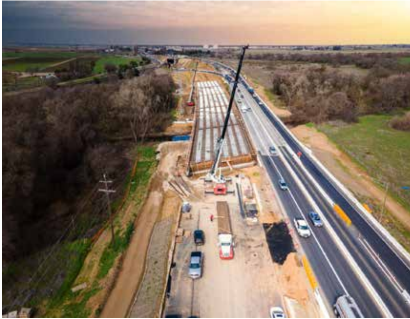
← Replacing six aging bridges with three modern spans required rerouting multiple lanes of traffic while avoiding power lines and a high-pressure fuel line nearby. Photo provided by Granite.
