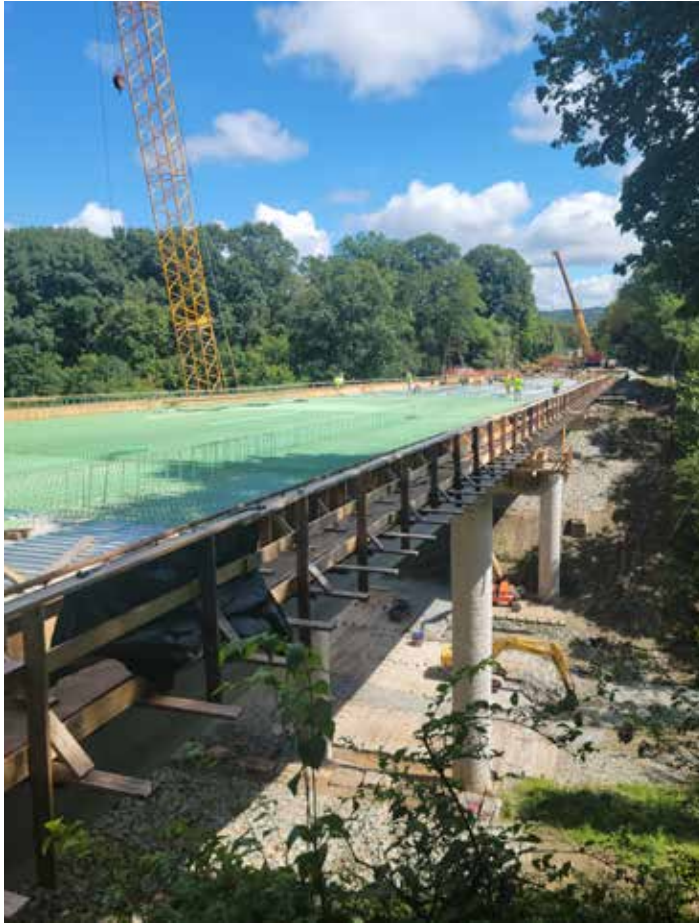
Workers prepare the bridge deck of the new Fern Hollow Bridge in September 2022 ahead of the concrete pour. Photo courtesy of HDR, Inc.
