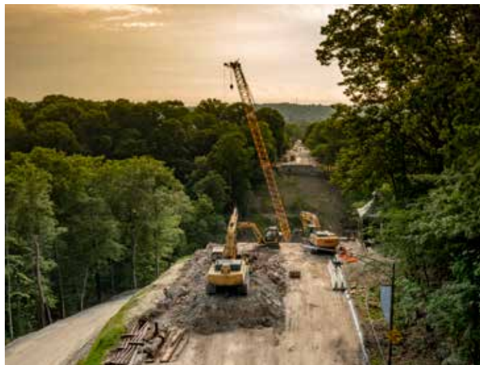
West approach site preparation work takes place on the Fern Hollow Bridge in Pittsburgh, early June 2022. Photo courtesy of HDR, Inc.
