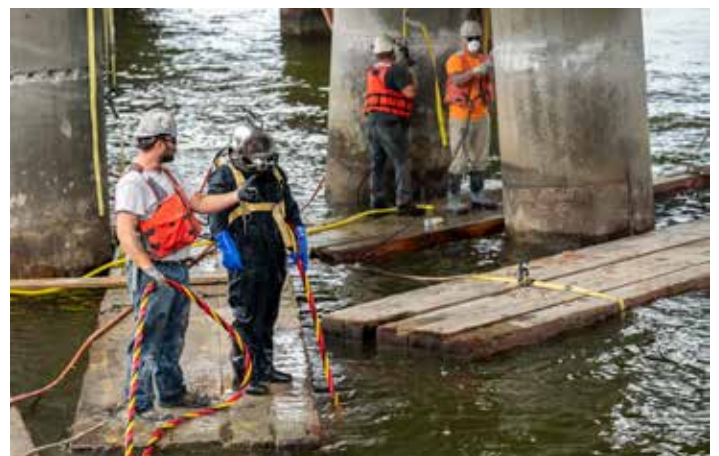
Dive crews repair bridge piers in New Jersey. Photo courtesy of Mount Construction.
